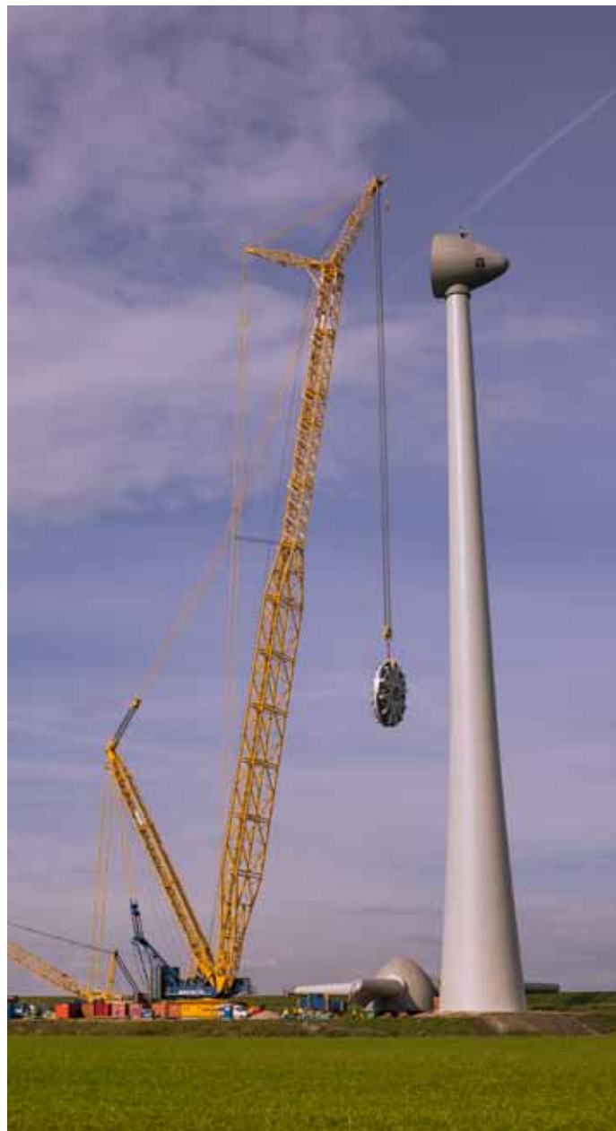
The CC 8800-1 with the BoomBooster extension arm system can take on loads of up to 3,200 tonnes.
