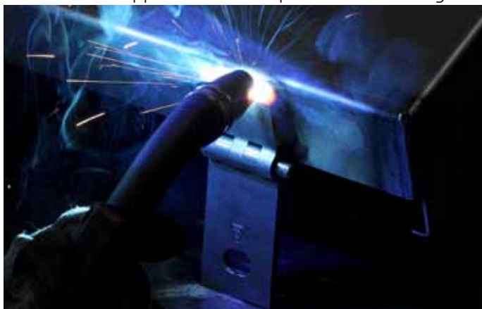
Photo 5: If robot welding is not economical due to the order quantity or component geometry, the parts are welded by hand.
