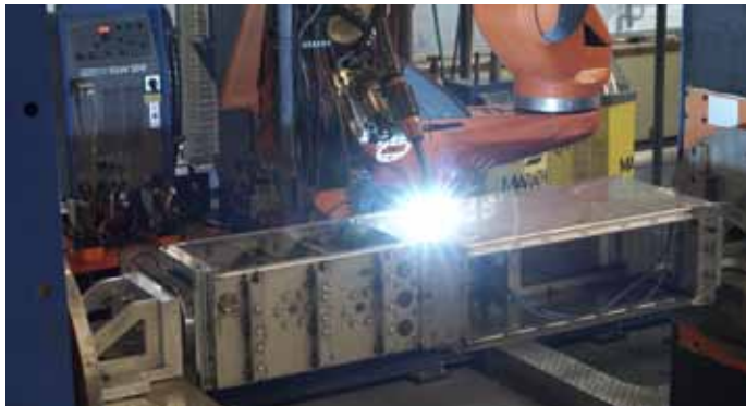
Photo 1: Driescher-Wegberg uses the CLOOS robot system to weld housings of switching systems.
